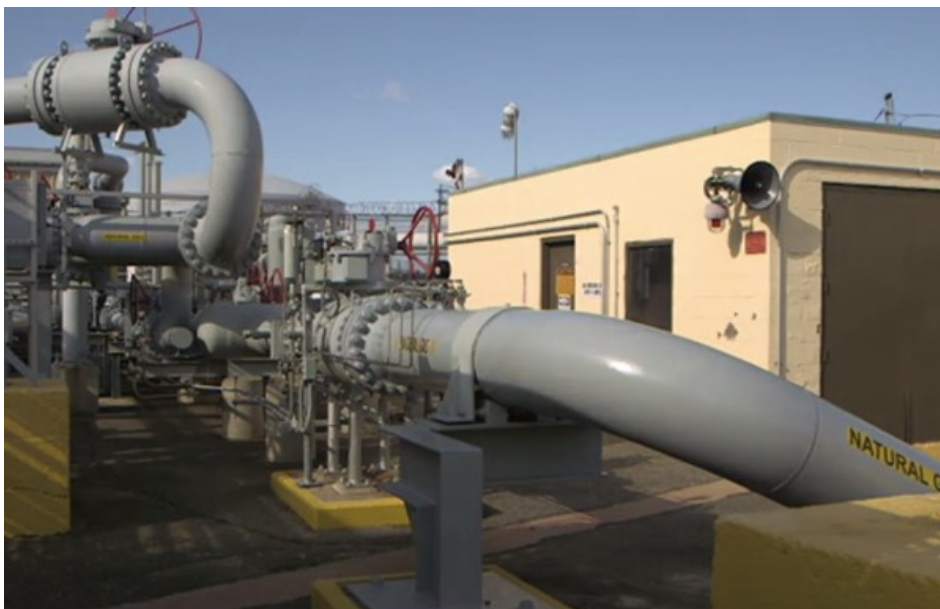
Distrigas Terminal | ENGIE
